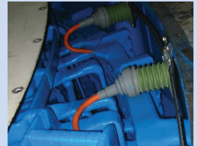
Installed Iris Power PDA couplers within a hydro generator
