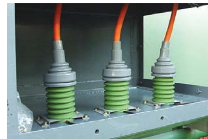
Installed Capacitive Couplers
